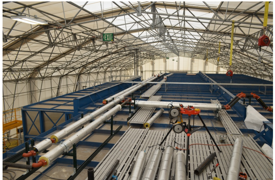
Cooling System for Nitrate Salt Drums
